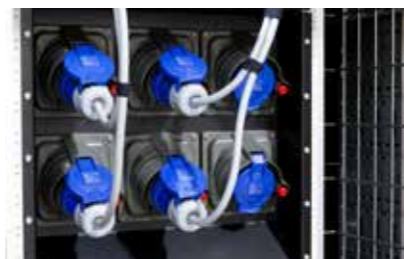
MatrixCube: Power distribution
